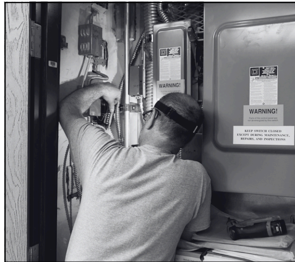
Fire and Life Safety performing routine maintenance and asset updates at the 108 River Street Building
