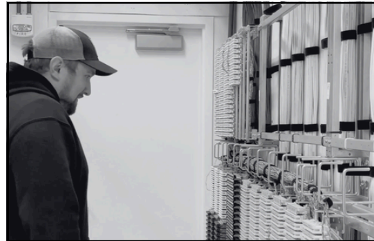
A Building Operations and Maintenance team member inspects equipment as part of preventative maintenance
