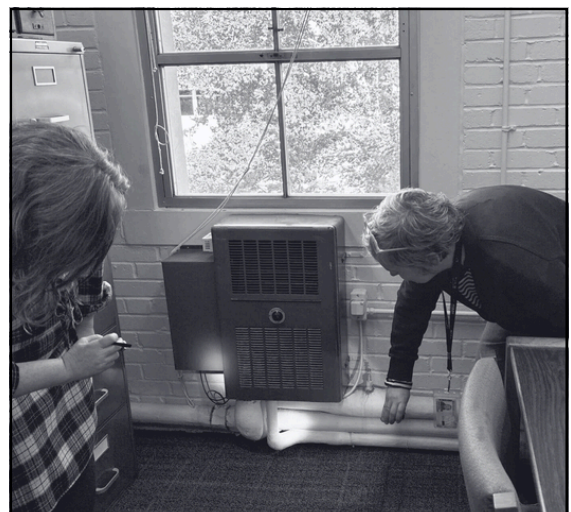
Building Operations and Maintenance teams collaborate with Main Library staff during the annual cooling-to-heating switchover
