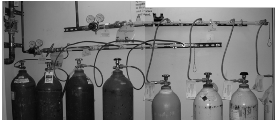
Figure 2: Existing reserve cylinder room at UIHC
