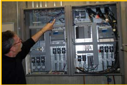
Photo: Energy Hawk Carl Stieglitz explains the temperature control system in the Lindquist Center building.
