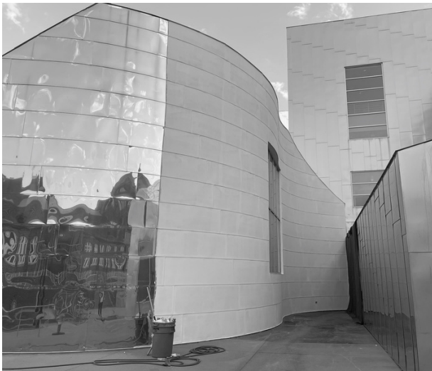
Exterior of the Iowa Advanced Technology Laboratories with the temporary coating applied following repairs
